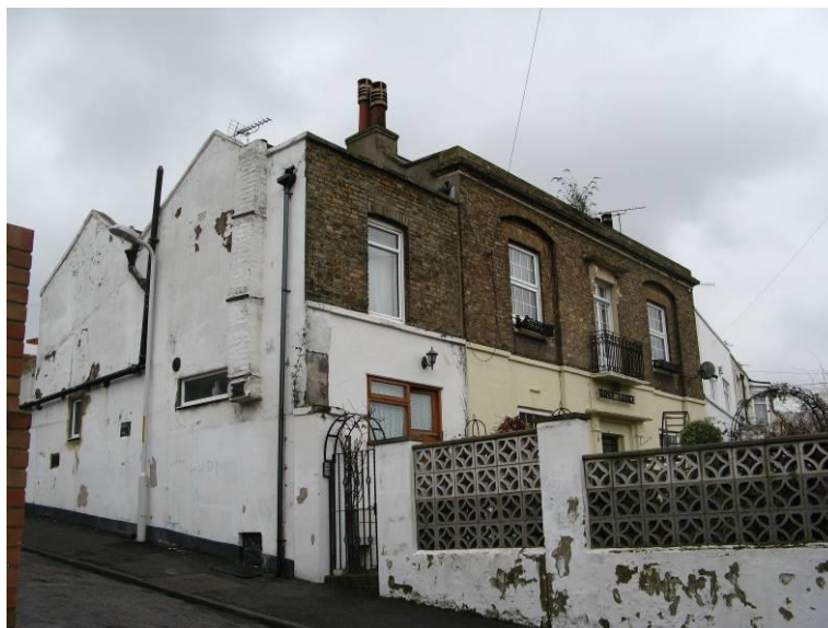
Rose Lodge is in urgent need of improvements
